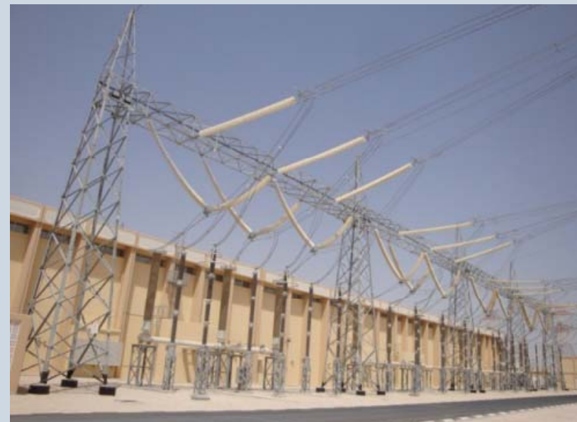
Faza VII - NCC Dalekovodi - 400kV 800MVA Abu Naklah Super
